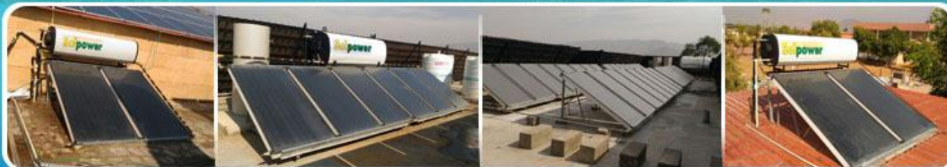
Solpower SWHS at The Westin, Pushkar, Rajasthan
